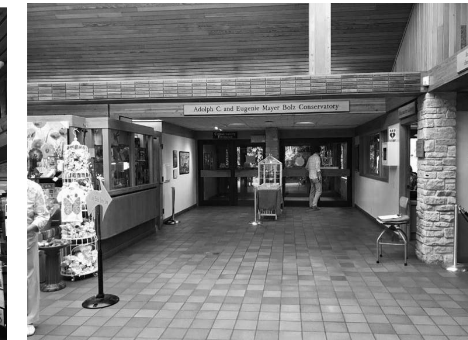
EXTG LOBBY LINK TO CONSERVATORY DOORS: ACT TILES TO BE REPLACED, GRID TO REMAIN. WOOD CEILING TO REMAIN AS IS.
