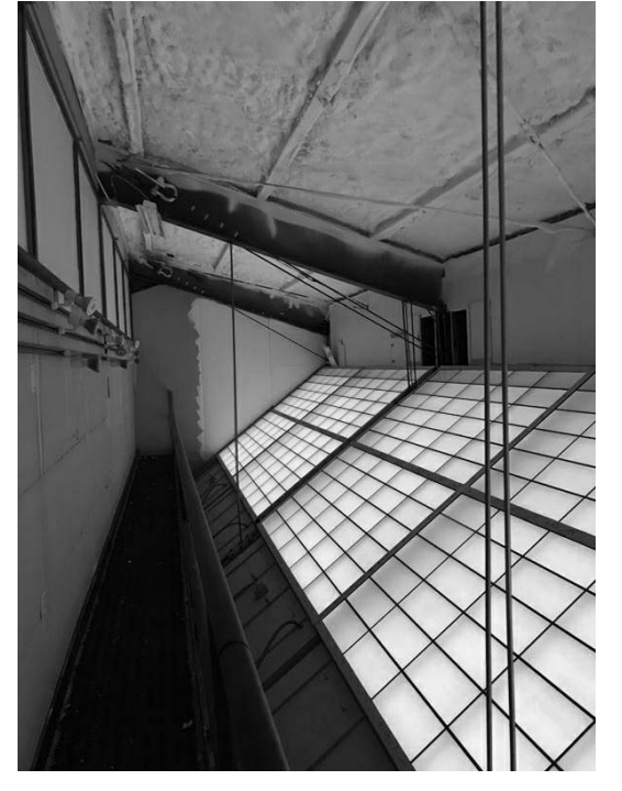
EXTG COMMONS CEILING VOID AND CATWALK: EXTG CEILING TO REMAIN, AND PATHWAY FOR UTILITIES BETWEEN HEADHOUSE AND LEARNING CENTER.
