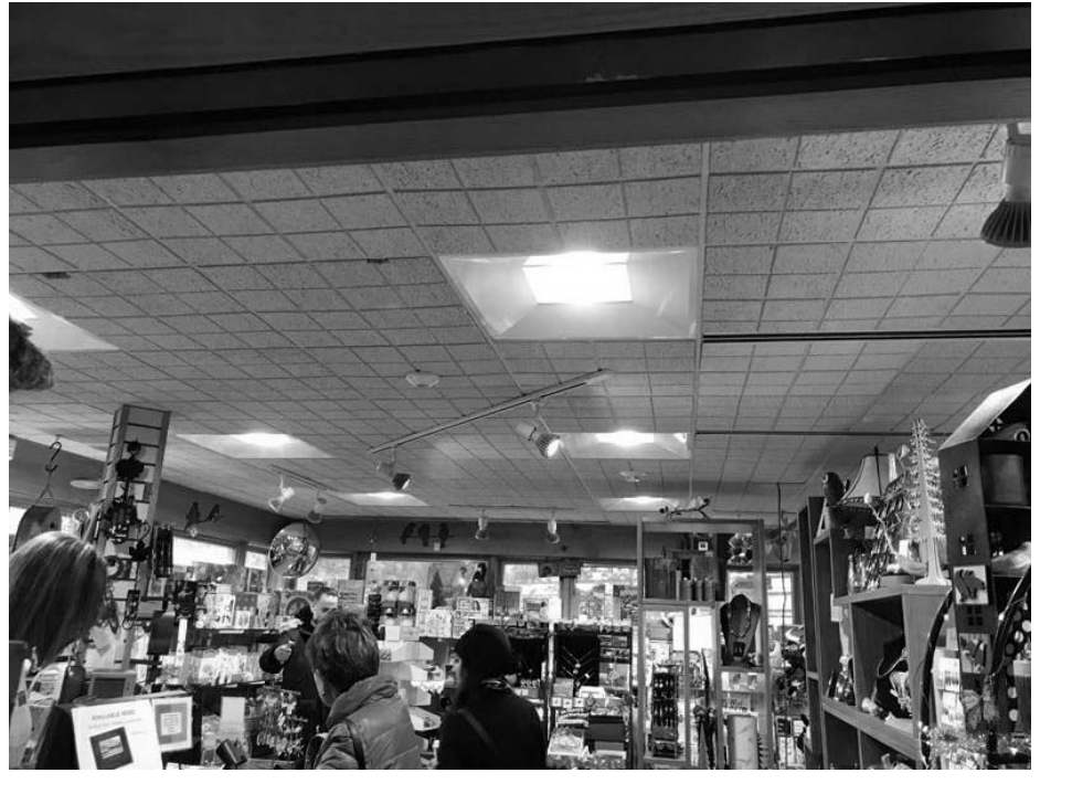
EXTG GIFT SHOP CEILING: EXTG CEILING TILES TO BE REPLACED, GRID TO REMAIN.
