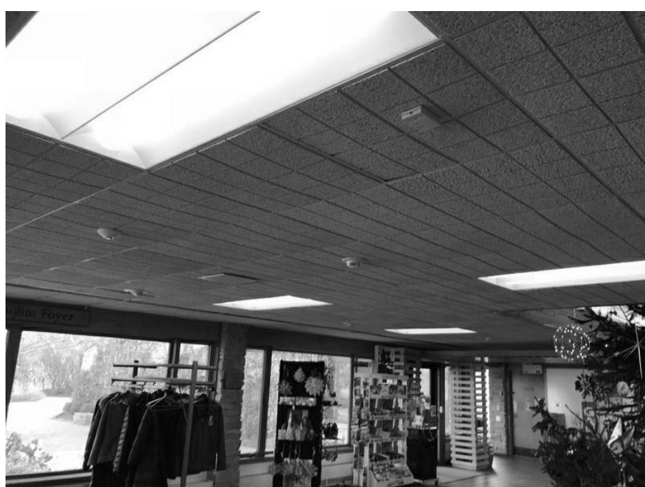
EXTG LOBBY WINDOWS AND DOORS TO GARDEN: EXTG CEILING TILES REPLACED, GRID TO REMAIN.
